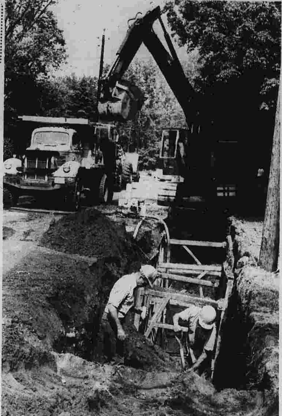
Workmen shore up a trench in Hillard St., looking east from Broad St. to Bilyeu Rd. The trench will hold a 42-inch pipe, expected to correct the storm-drainage problem prevalent for years at Broad and Hillard Sts. The work is being done by the Gem Paving Co. of Newington, under a contract estimated at over $100,000. The plan calls for routing the storm water via Bilyeu and Fleming Rds. into the Hockanum River. (Herald photo by Pinto)
